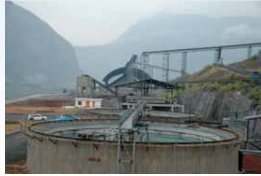
Xiluodu Majiaheba Aggregate Processing Wastewater Treatment System
